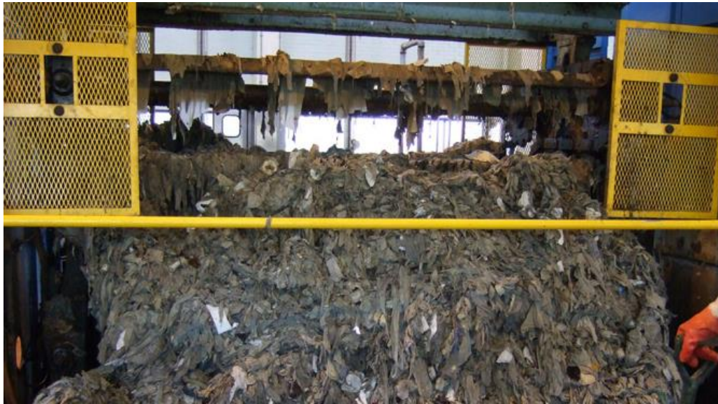
Figure 3-9: Refuse collected on wastewater treatment inlet screens 1
